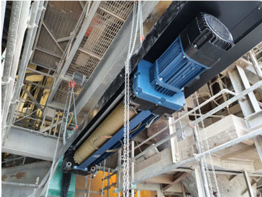
10-tonne SWL electric-powered wire-rope hoist unit lifted into final position at a 60m height by Hoist & Winch Ltd.
