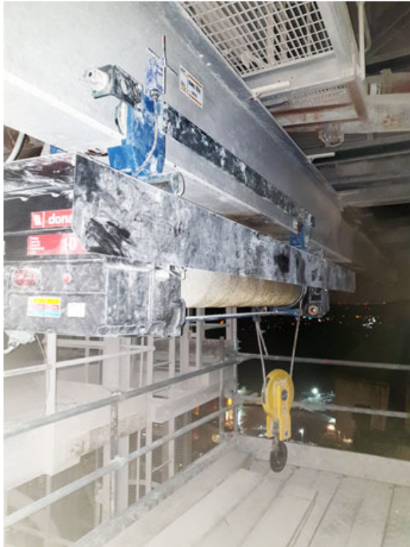
Wire-rope hoist in final position after installation and test by Hoist & Winch Ltd.
